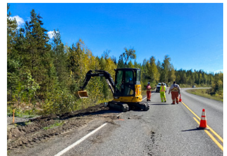
Right: CityWest fibre placing crew pushing fibre optic cable through plastic conduit along the edge of the pavement at depth of approximately one metre.
