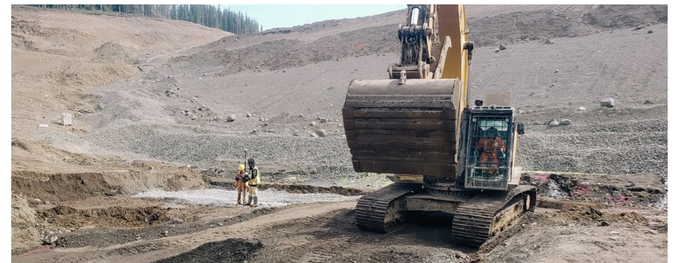
Below: TNDC crew and equipment at work on the Red Chris TIA project.
